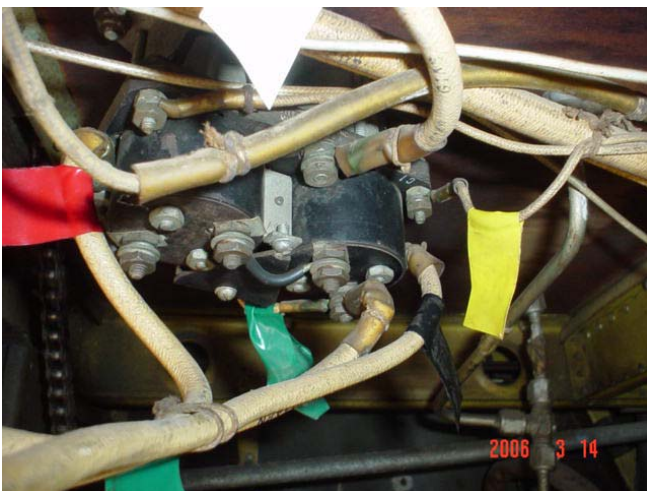
Old dynamic brake relay before removal...
