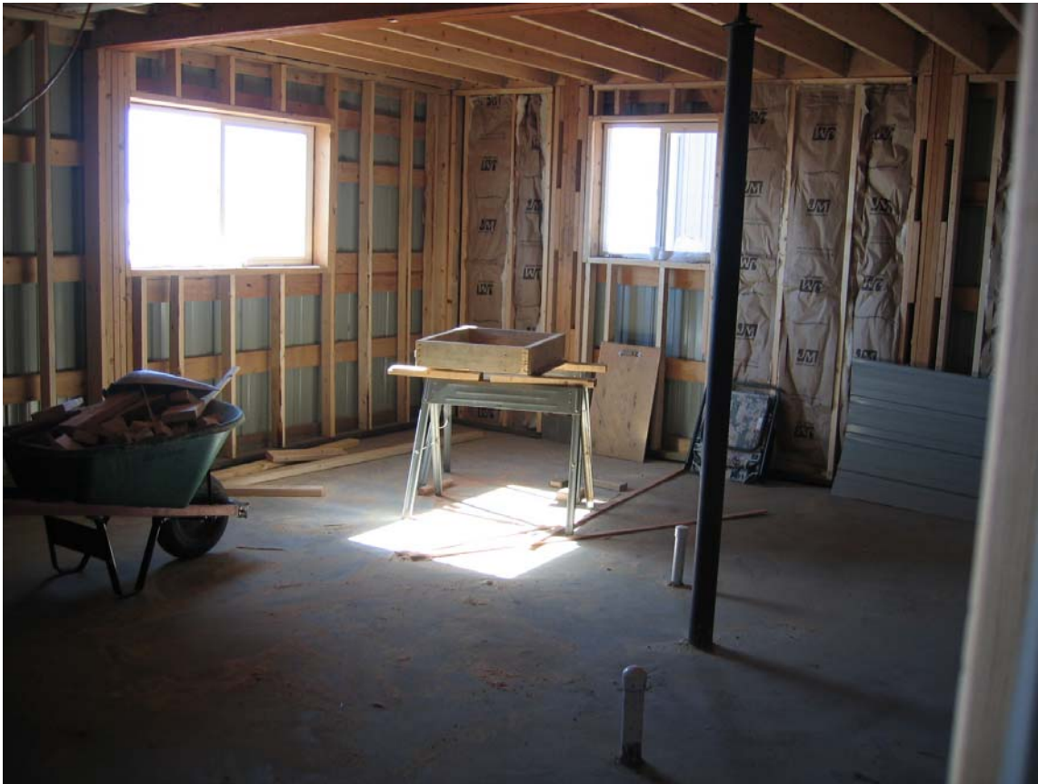
Pictured is interior of the snack bar area located in the southwest corner of the hangar, having two windows facing the south and west. This room will have an "L" shaped bar, and small kitchen. Picture was taken facing southwest.
